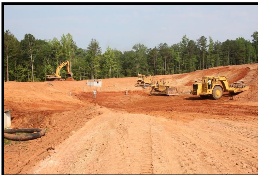
Figure 3: Construction of a stormwater retention pond, Athens-Clarke County. Photo by Rob McDowell, University of Georgia.
